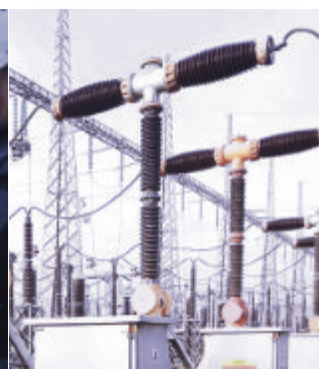
CORONA, PARTIAL DISCHARGE DETECTION
